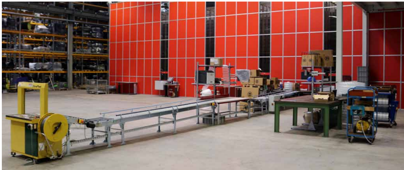
Noticeably faster processing right from the start: the automatic small parts warehouse
