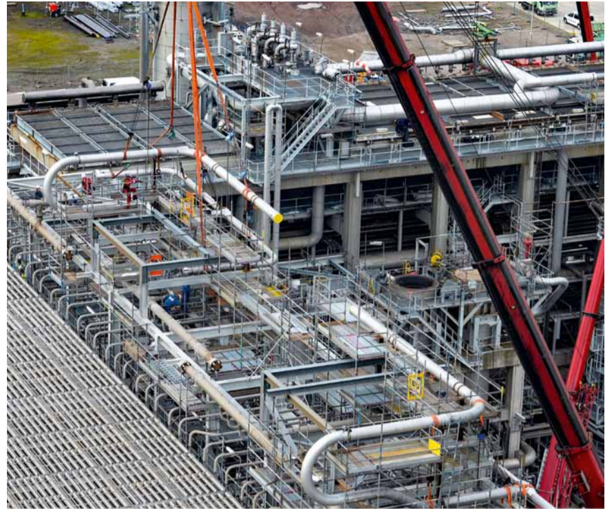
A real eye-catcher: the hydrocracking unit for Shell Pernis
